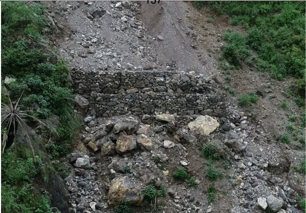
Photograph 9 - Retaining structures provided in the course of nallah downstream mining site
