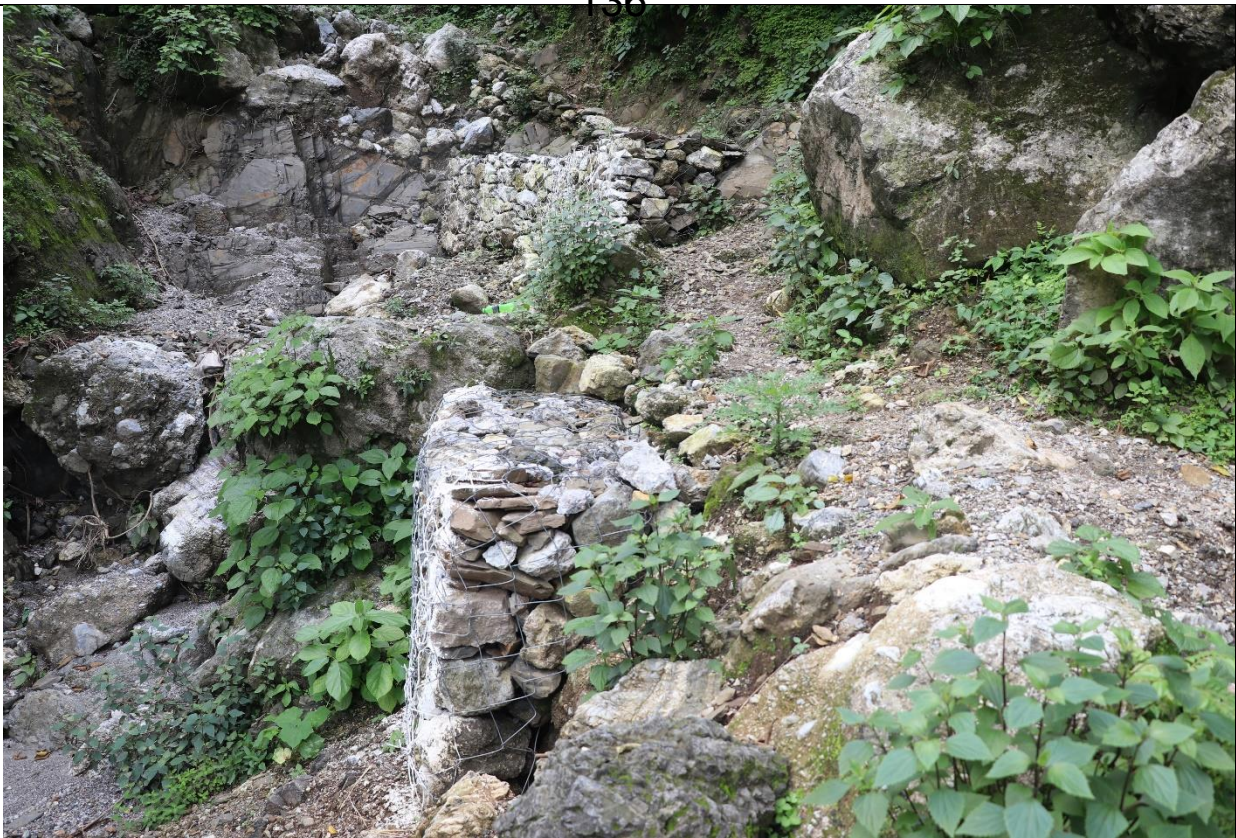
Photograph 7- Retaining structures provided in the course of nallah downstream mining site
