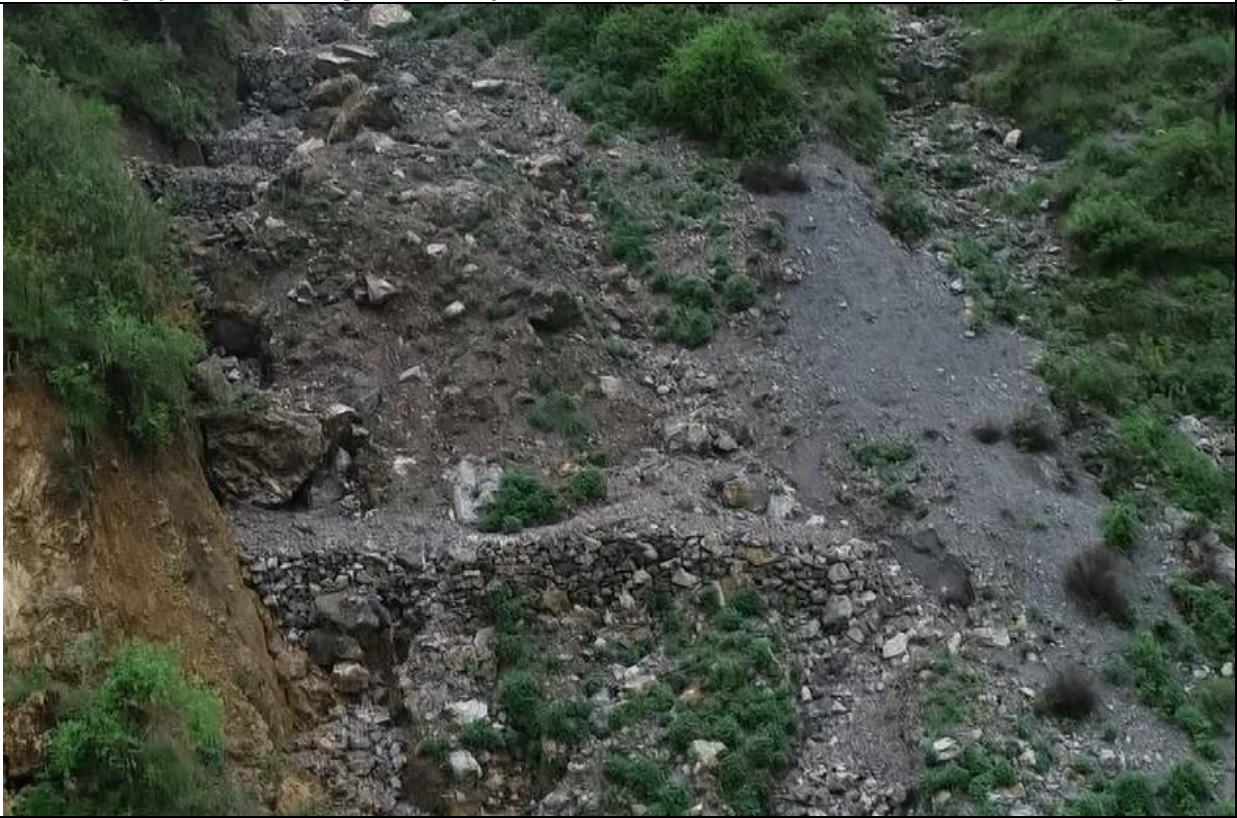
Photograph 10 - Retaining structures provided in the course of nallah downstream mining site
