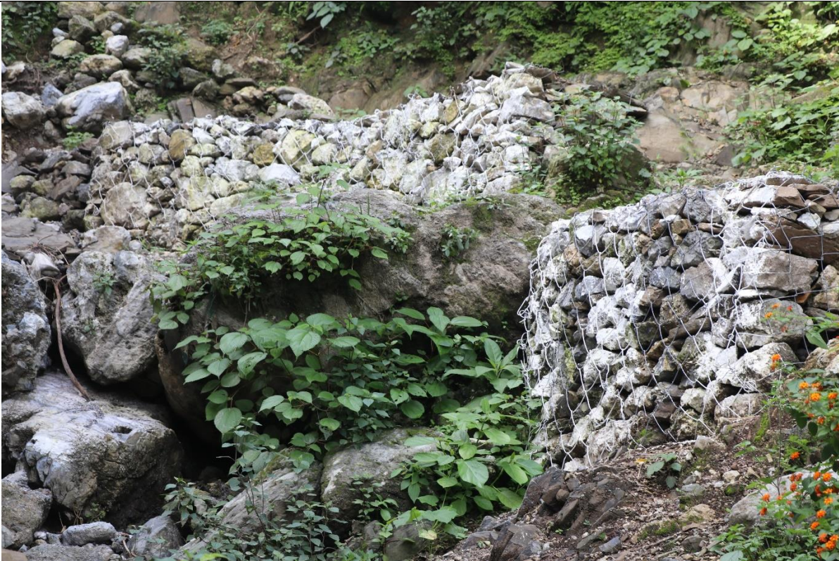
Photograph 6- Retaining structures provided in the course of nallah downstream mining site
